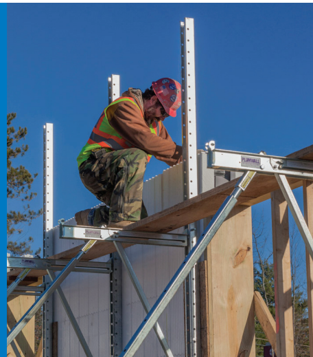
PHOTOGRAPHY BY CHRISTOPHER BARNES A construction worker installs an insulated concrete form at the new medical office building under construction for St. Joseph's Healthcare in Bangor. Consigli Construction introduced the innovative ICFs for the new 22,000-square-foot building.
